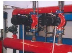
New energy-efficient circulation pumps
