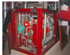
New CHP plant
