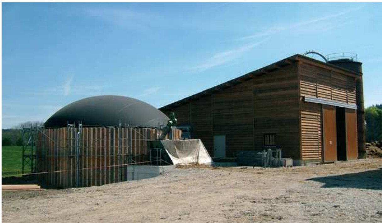
The biogas plant at the end of the construction phase, May 2007 © Suisse
